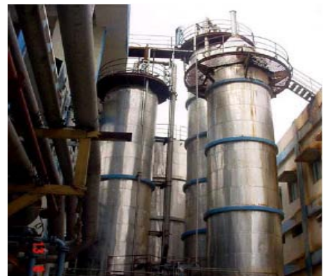
Figure 4.1 Oxygen De-lignification Tower
